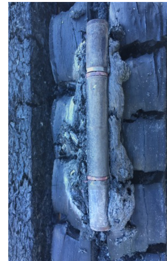
Intumescent around hinge
