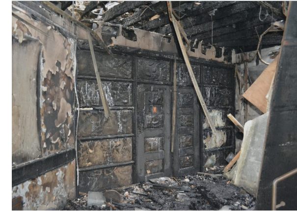
Internal side of fire door after fire
